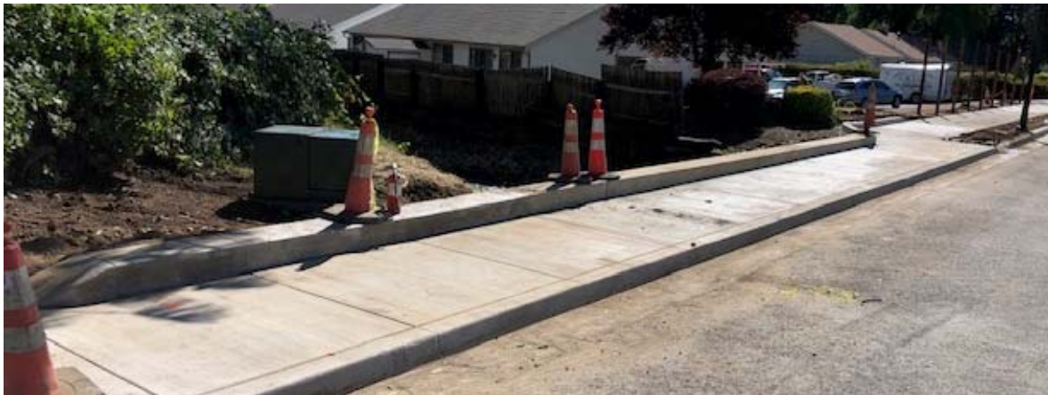
The culvert over the Buchanan channel was completed, and the bypass removed.
