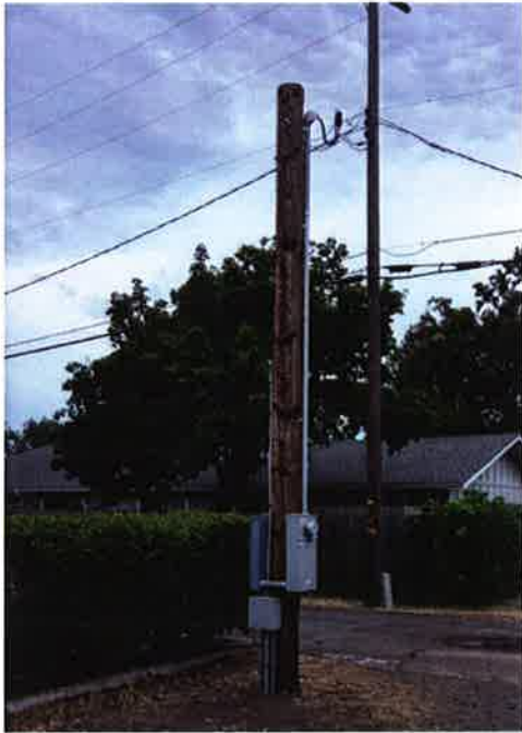
Pacific Electrical Contractors installed new electrical service for the Old Fire Station and Main Street lights.
