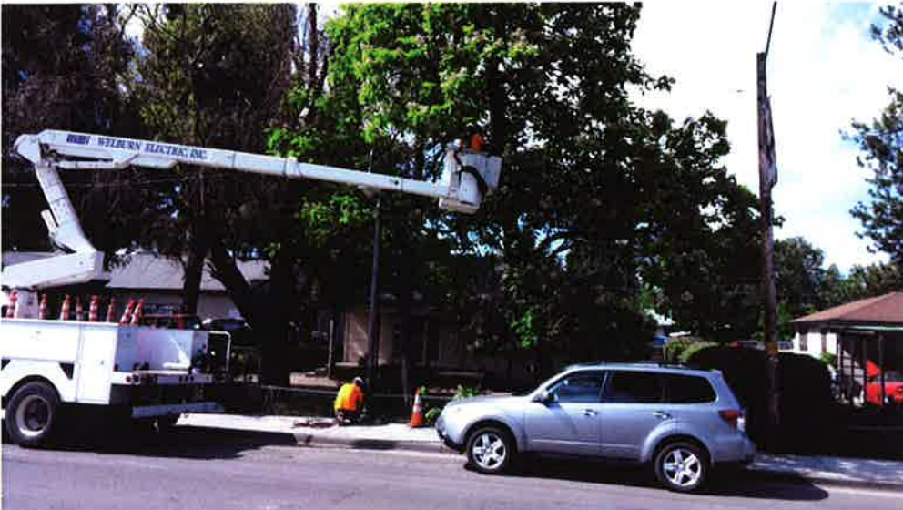
Welburn Electric installed three lights on Loto Street. The lights were supplied by the City.
